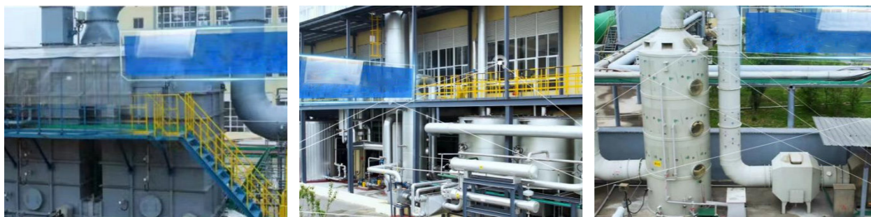
▲ Waste gas treatment system
